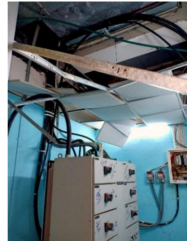
Pic 3.12: Collapsed false ceiling of the Electrical Unit at ground floor of the Auditorium
